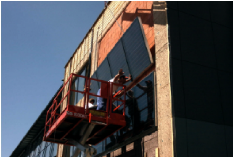
Figure 16: Mounting of test collector on a brick wall of the south-west façade of an office building with the help of a crane. 25 m 2 collector area (5 m x 5 m)
