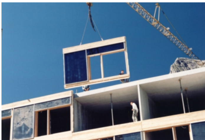
Figure 3: Construction of a hotel in Austria with façade-integrated collectors. A high level of pre-manufacturing is possible
