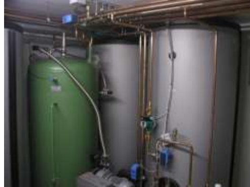
Figure 3.3.3: Storage tanks installed (from left: water reservoir containing evaporator/condenser heat exchanger, one of two silica gel tanks containing spiral heat exchanger, conventional energy storage tank, source: AEE INTEC, Austria.
