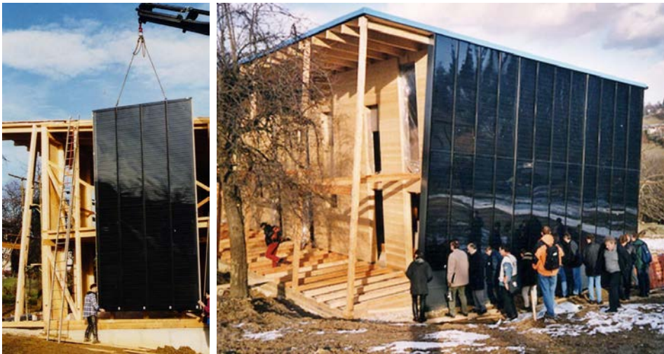
Fig 3.1-6: Two-family dwelling, Austria, 2001. Project management I. Bergmann, W. Weiss AEE-INTEC, AKS Doma façade collectors (credits AEE INTEC).
