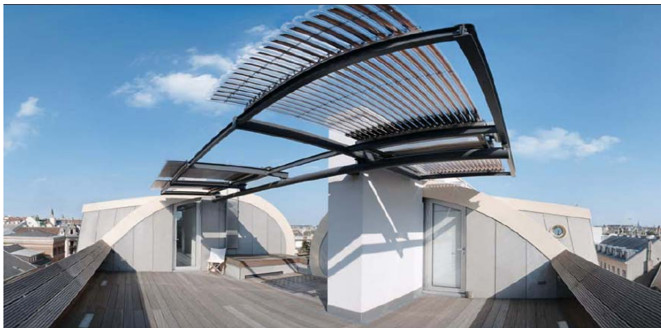
Fig.3.3-5: Evacuated tubes collectors used as deck sun shading. RaU Architekten, Vienna. Credits: RaU Architekten.
