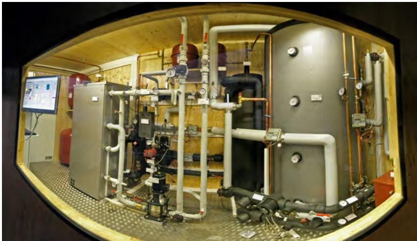
Figure 1: Installation at the office building of the Company SOLID in Graz, Austria (17.5 kW Yazaki chiller WFC 5). (Source: SOLID)
