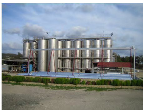
Figure 3. Solar cooling installation at a winery in Tunisia.
