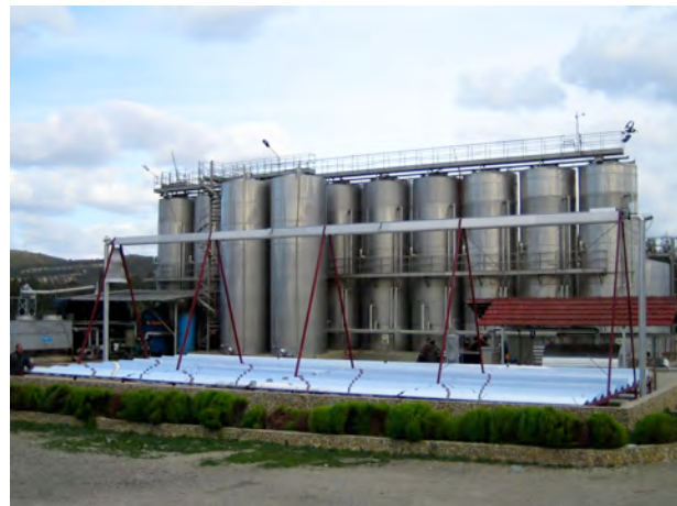
Figure 3. Solar cooling installation at the winery in Tunisia. In front: the Fresnel collector; the cooling of the wine storage tanks, shown in the background, is supported by the chiller, connected to the Fresnel collector.
