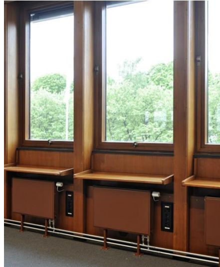
New radiators mounted under the windows on protected exterior walls
