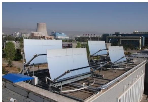
Figure 8: Demo system of Sun Oyster on a flat roof in Zhangjiakou, China (sunoyster.com)
