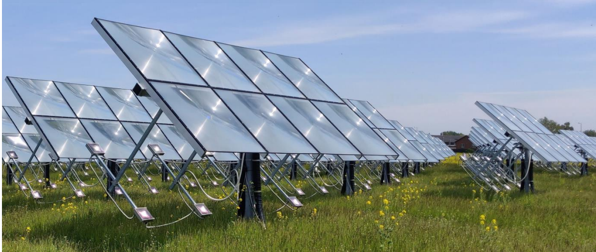
Figure 24 Photo of Fresnel lenses, Heliac in Denmark (Jensen, Sifnaios, Caringal, Furbo, Dragsted, 2022)
