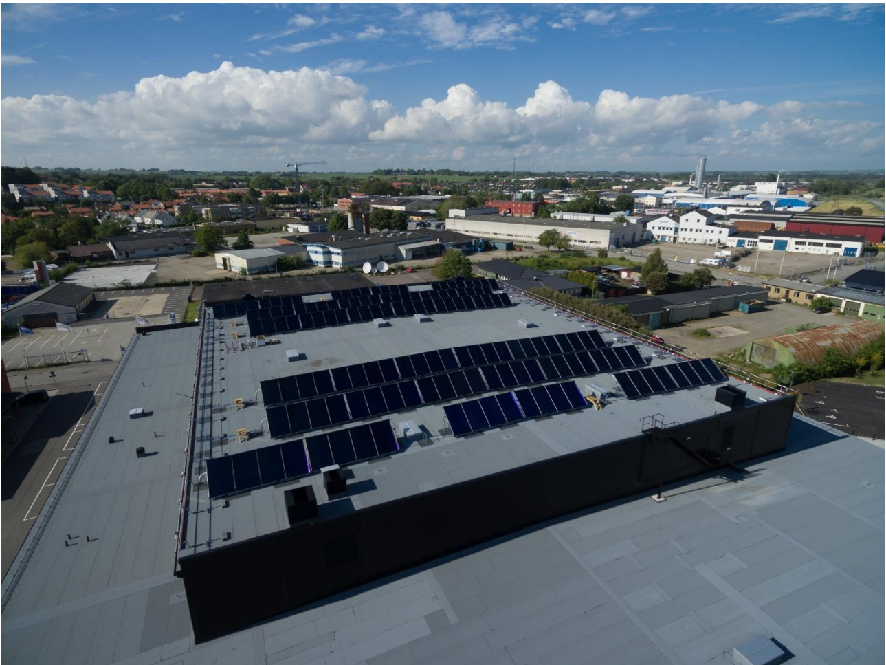
Figure 18. Rooftop-mounted ST collector field Ystad (Sweden)
