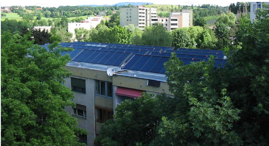
Figure 16. Rooftop-mounted ST collector field in Berlinerring (Graz)
