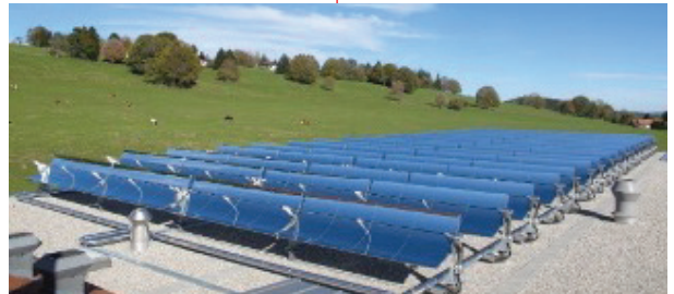
Emmi Dairy Saignelégier in Switzerland uses parabolic trough collectors to generate steam for different dairy processes. (Source: NEP Solar AG / SHIP database, http://ship-plants.info/ )
